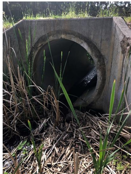
Photo 8 –Upstream end of culvert at Deep Creek crossing. Pipe diameter is approx. 1.5m.
