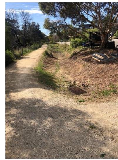
Photo 11 – Stormwater infrastructure adjacent to the walking track at the bottom of Tea Tree Rise.
