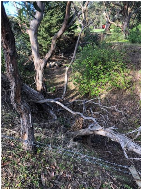
Photo 1 – Tributary input to Deep Creek (looking upstream). Gully is developing and deepening in response to lower bed level in Deep Creek.
