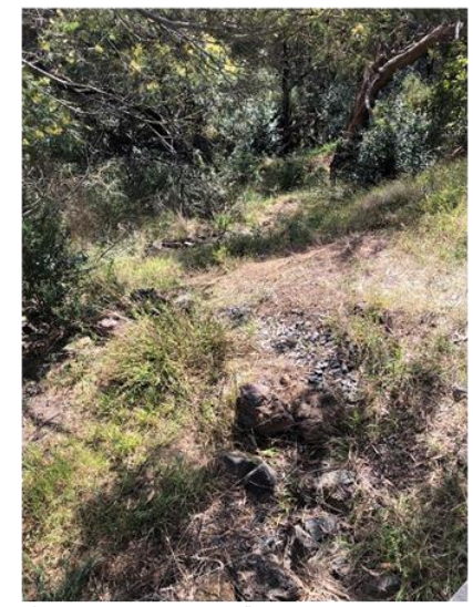
Photo 12 – Stormwater overflow structure entering Deep Creek at the bottom of Tea Tree Rise.
