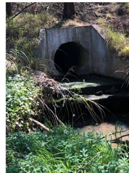
Photo 15 – Downstream end of stormwater inlet to Deep Creek (upstream of Fisher Street). Pipe diameter is approx. 1.0m.
