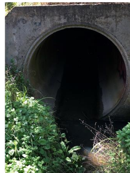
Photo 16 – Upstream end of culvert along Deep Creek at Fisher Street crossing. Pipe diameter is approx. 2.0m.
