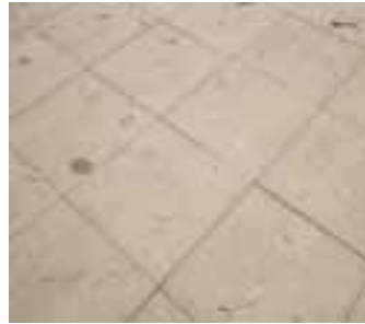
Concrete slabs are generally cracked, marked and in poor repair.
