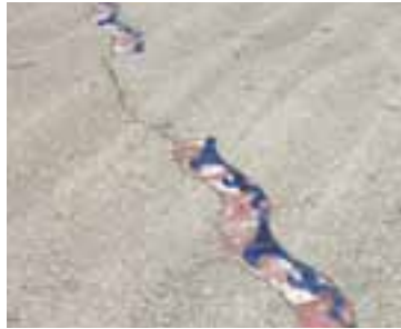
Concrete slab with exposed aggregate is used within the majority of the streetscape. Inlaid decorative tiles are in poor condition.
