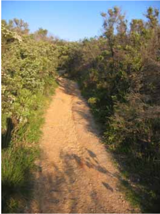
The Lighthouse Heritage Trail is the precinct's main pathway. The gravel surface limits access for people with disabilities and is erosion prone. A better path would encourage visitors to experience the precinct on foot
