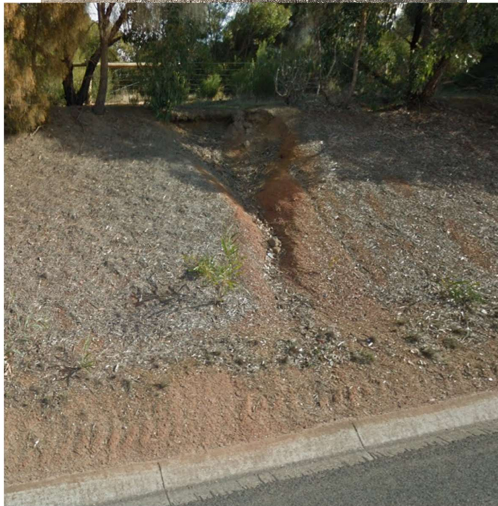
Figure 2 – Photos external to the east side of site of existing erosion from runoff from site
