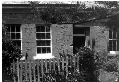
Figure 4: Former Presbyterian Manse, part of north elevation, 10 November 1985. Source: J.T. Collins, La Trobe Picture collection, State Library of Victoria, accession H90.110/1166.
