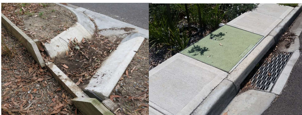
Figure 16 Examples of sediment traps located at the bioretention inlet zone.
